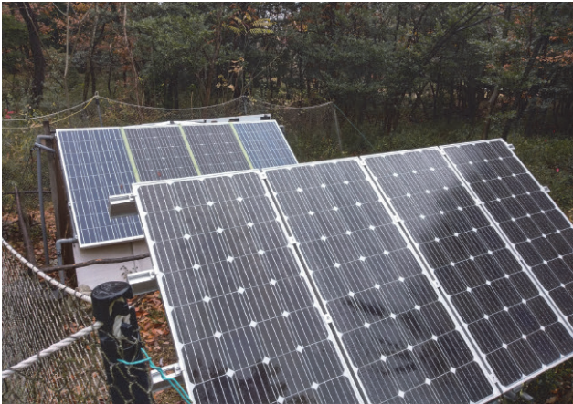
Solar battery panels powering the on-site equipment
